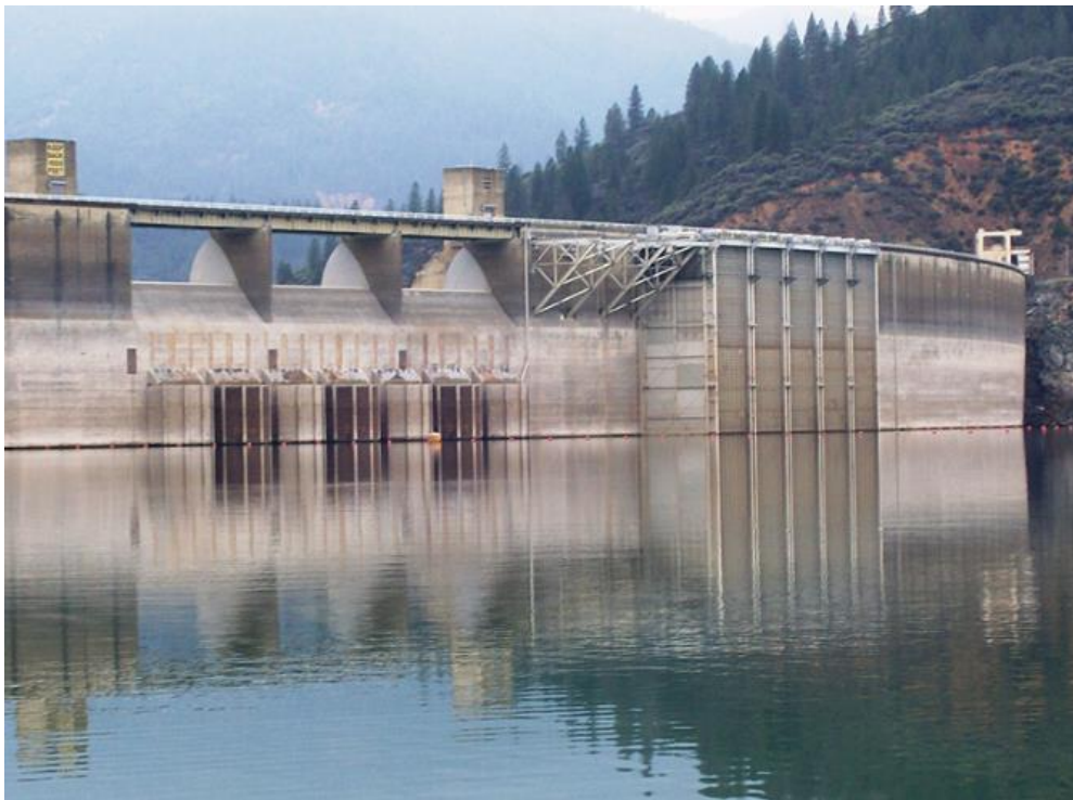
Figure 22. Shasta Dam (looking downstream) showing spillway, river outlet trash racks, and TCD.
